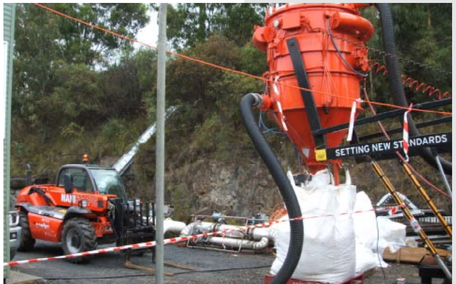
Photo (bottom) - All removed decanted mater was transported to and disposed of at the Lucas Heights WSN waste disposal facility.
