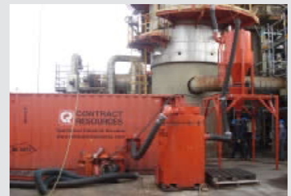
Photo - Vacuum Unit set up on site at Repsol, La Plata
