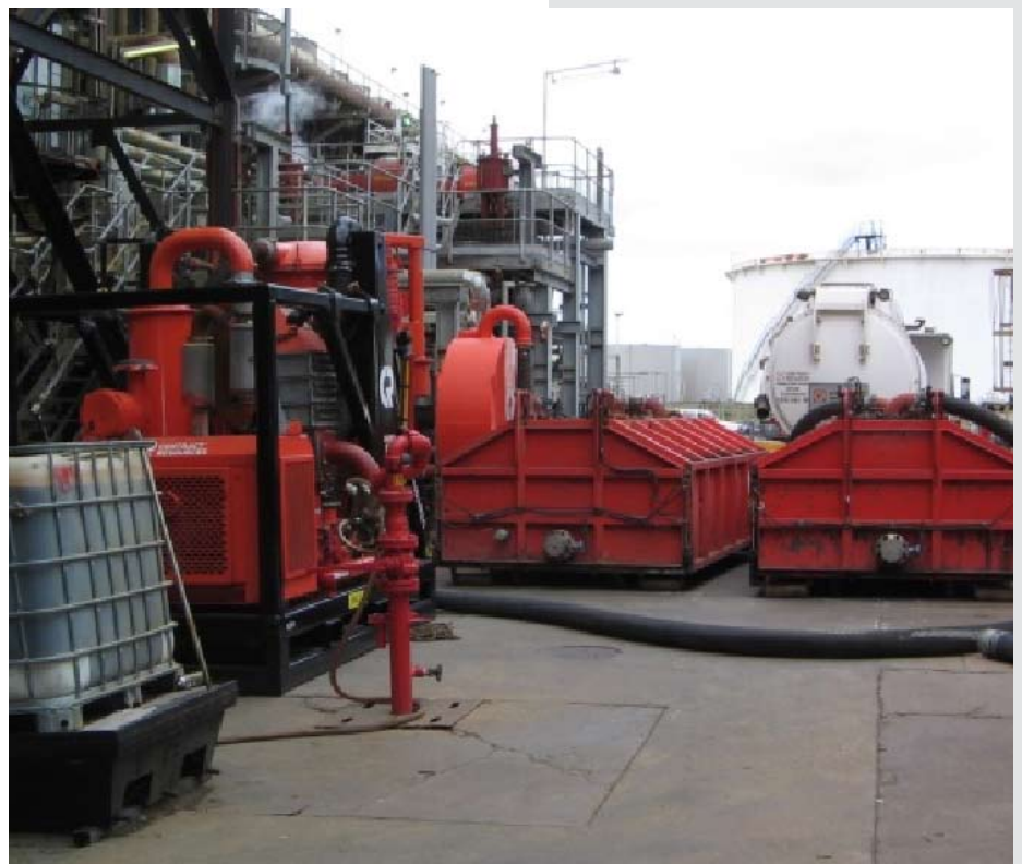
Photo - Vacuum units at base of R & R
