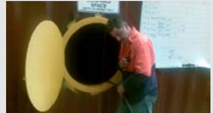
Attila Veroes acting as stand-by person, maintaining communication with persons inside confined space
