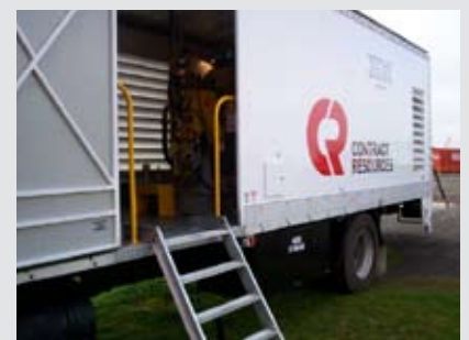
HP044 - Step into main engine room
