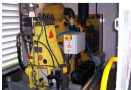
HP044 - Pump unit
