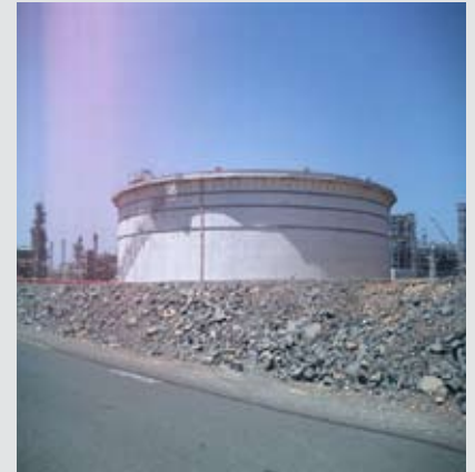
Photo - The Condensate Tank 2t 3301 at the Karratha On shore Gas Treatment Plant.
