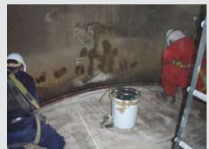
Photos - Crew doing mechanical isolations & internal repairs at the BP Bulwer Island facility
