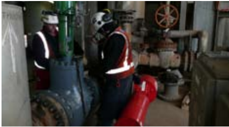
Photo - M.McMahan and M.Bouma torqueing up flanges after the filtration unit was put into place.
