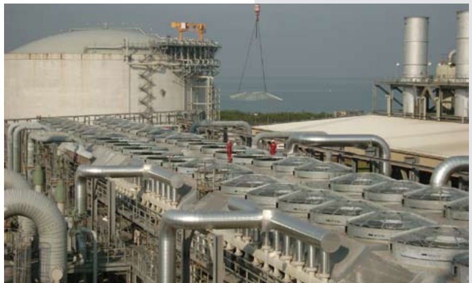
Photo - The CR crew installed 90 Fin Fan covers with the use of Rope Access
