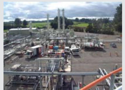
Photo - The Waihapa Production Station
