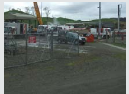
Photo - The Mangahewa Production Station
